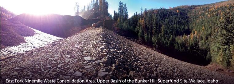
East Fork Ninemile Waste Consolidation Area, Upper Basin of the Bunker Hill Superfund Site, Wallace, Idaho
