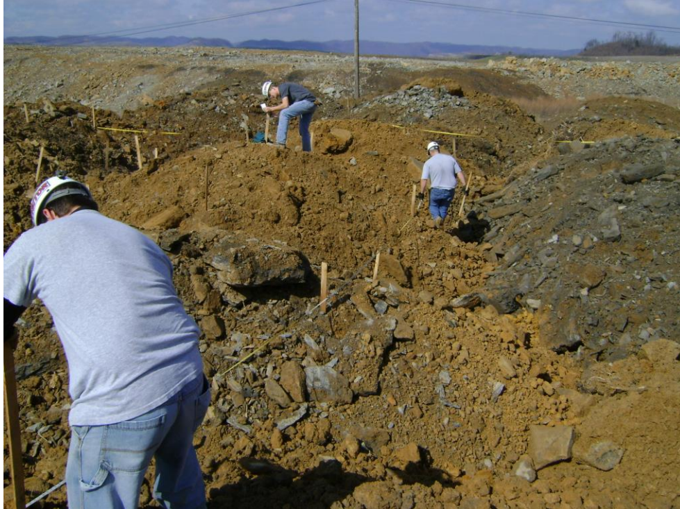
Figure 3. The 0.3-ha experimental area of brown sandstone and topsoil at Nicholas was constructed in 2009 and simply end-dumped with trucks.
