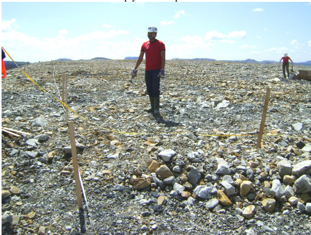
Figure 4. The 0.3-ha experimental area of gray sandstone at Nicholas was constructed in 2009 with primarily gray sandstone and some brown material, and graded and compacted by bulldozers.
