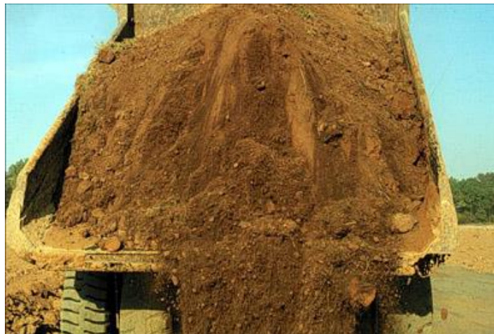
Figure 13. Rear-dump truck loaded and placing the equivalent of 36 in of subsoil and 12 in of topsoil on top of the load in one operation
