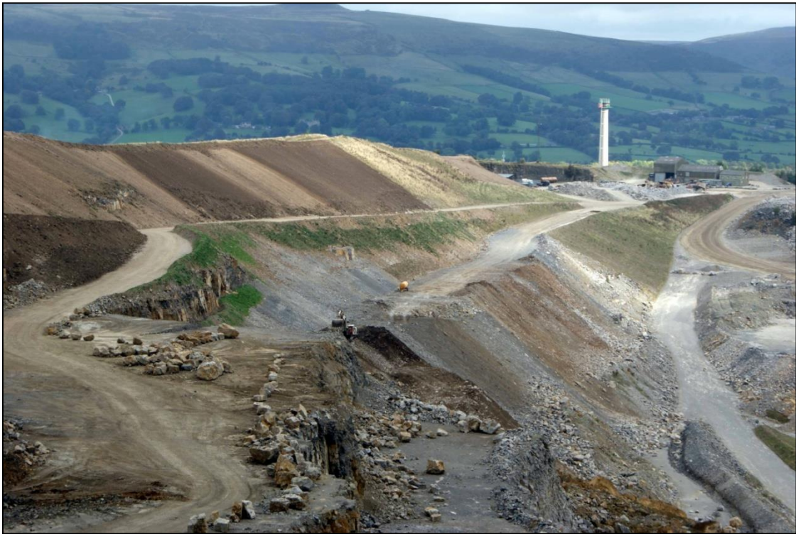
Figure 4. An example of rollover slopes being formed at the Hope Cement Works, Hope, Derbyshire, England. The technique was used in a progressive reclamation scheme to cover a number of benches where extraction has ceased.
