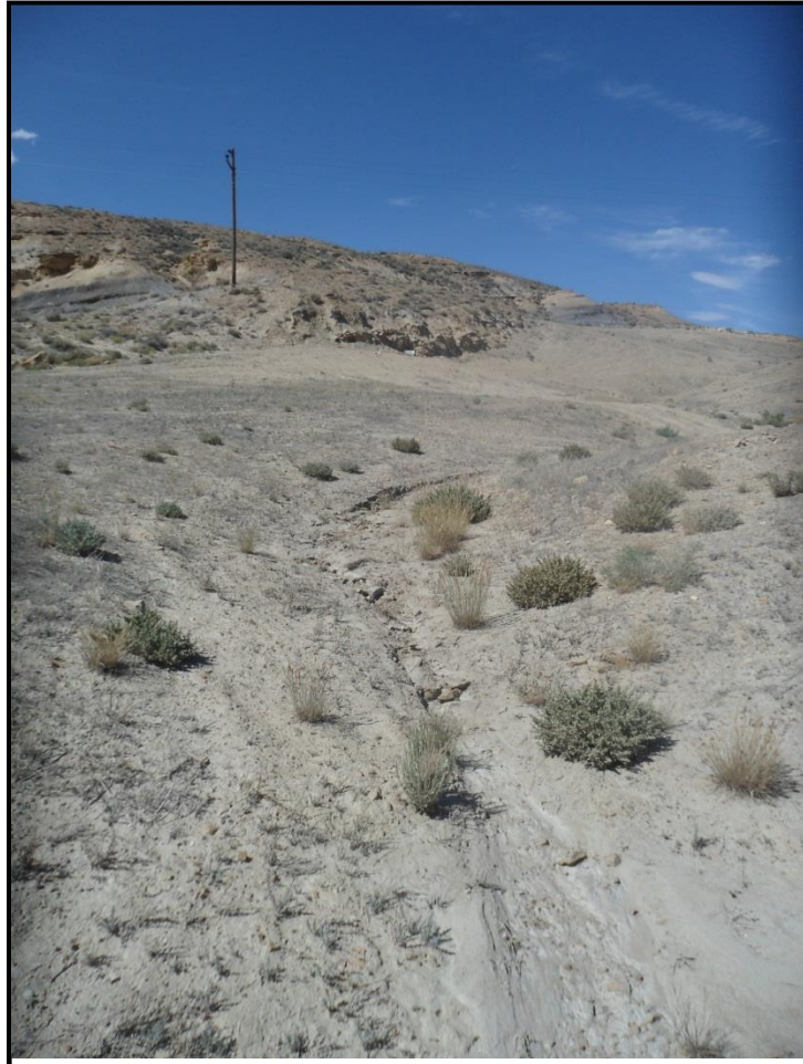
Figure 12. Reliance No. 11 North channel, looking upstream at a pilot channel forming in the channel bed. The channel is stable.
