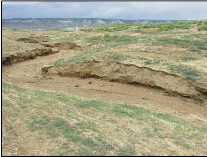
Figure 16. Channel bank cutting in 2016 at the confluence of the Lionkol Upper and Lower drainage. Repairs were made through a re-design of this section.
