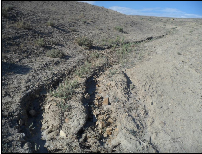
Figure 14. Reliance No. 3 North Spoils main channel failure, cutting through the point bar. The channel was repaired and widened.
