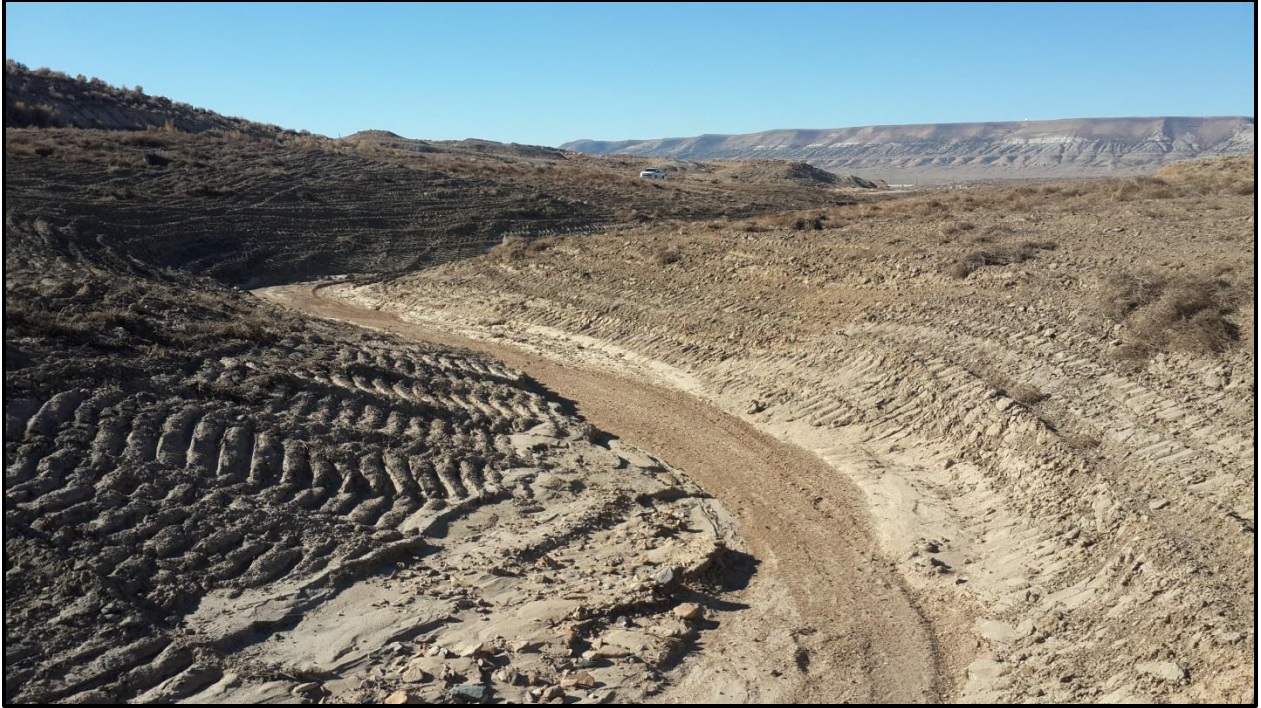
Figure 17. The regraded main channel of the Lionkol drainage after repairs in fall 2016. A storm event tested the channel shortly after the repairs were made.
