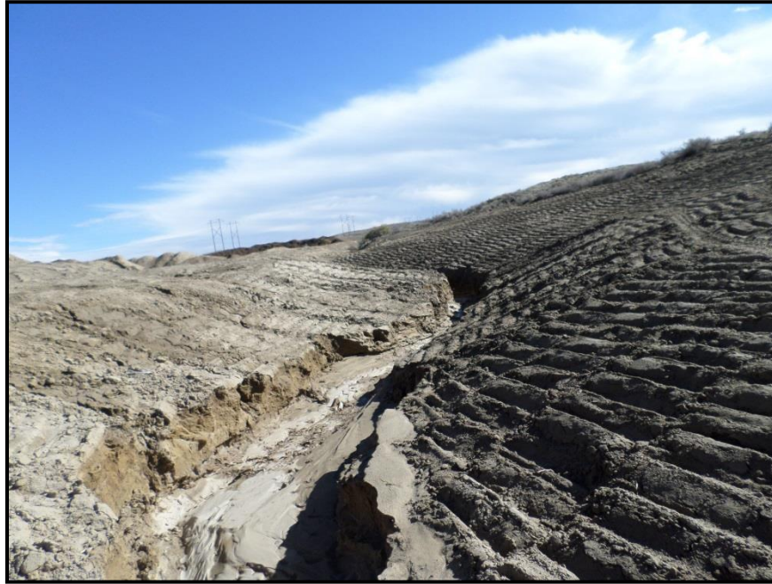
Figure 18. Lionkol West, Upper Reach. Channel erosion from storm events during construction.
