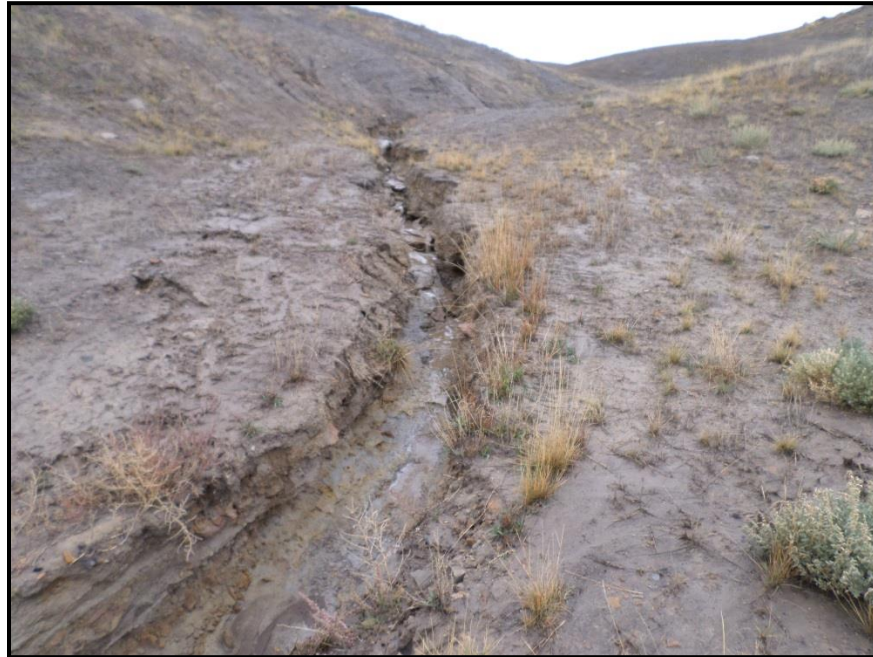
Figure 15. Lionkol North Main channel failure, incised to bedrock. The channel was repaired by widening the bed and sloping the banks.
